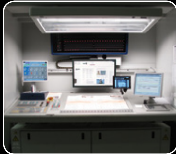
Custom-made control center housing.
